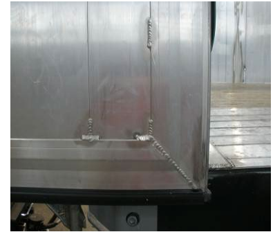
Side walls: Check the weld seams for cracks
